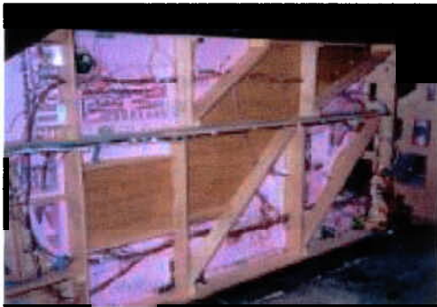
(Photo 1 - Bridges Canyon bottom of left-hand module.
